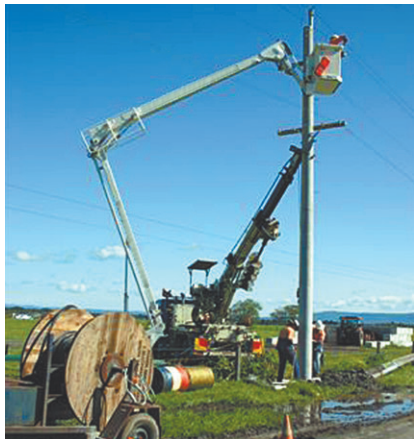
The team from South East Power Lines replacing old wooden power poles with new concrete poles to conform with current regulations in a rural subdivision
